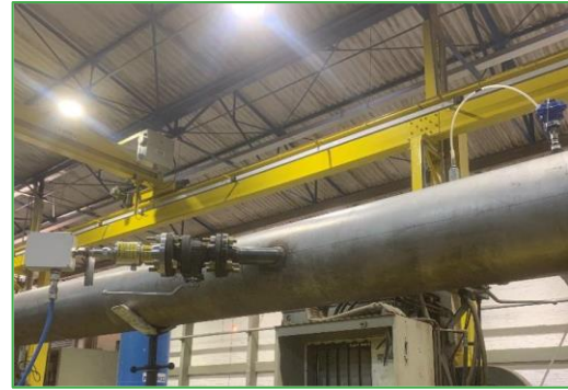
Fig 4. Fluenta transducers mounted on 12" pipe. Source: IPT.
