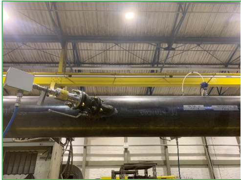
Fig 3. Fluenta transducers mounted on 16" pipe. Source: IPT.
